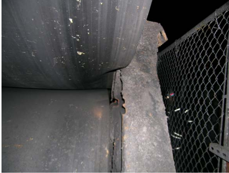
Figure 1. Evidence of belt misalignment.
