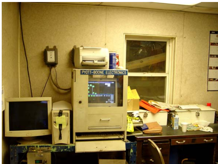
Figure 11. AMS in dispatcher's office located in Box Cut on surface.
