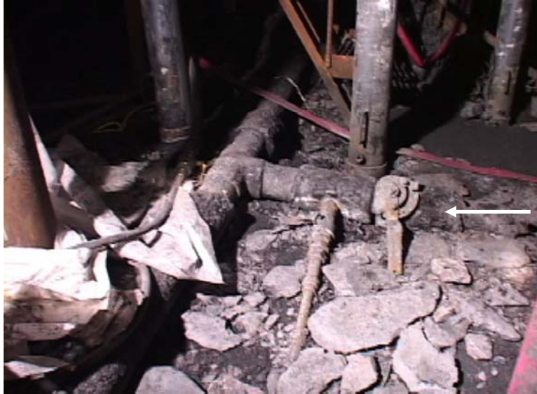
Figure 14. 4-inch water valve (found in “off” position)
