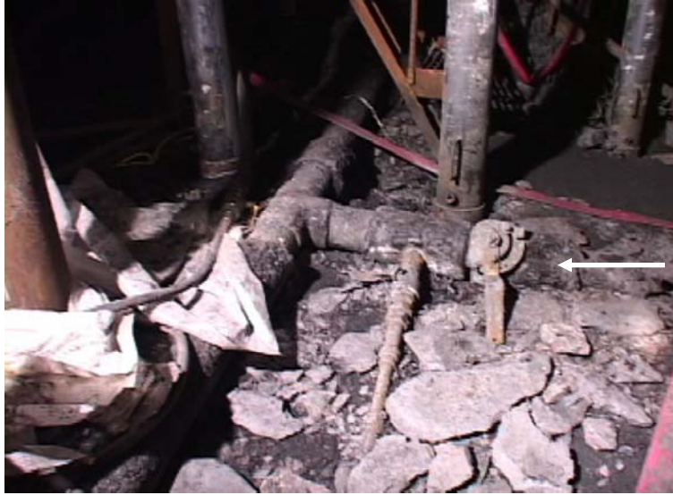
Figure 14. 4-inch water valve (found in “off” position)
