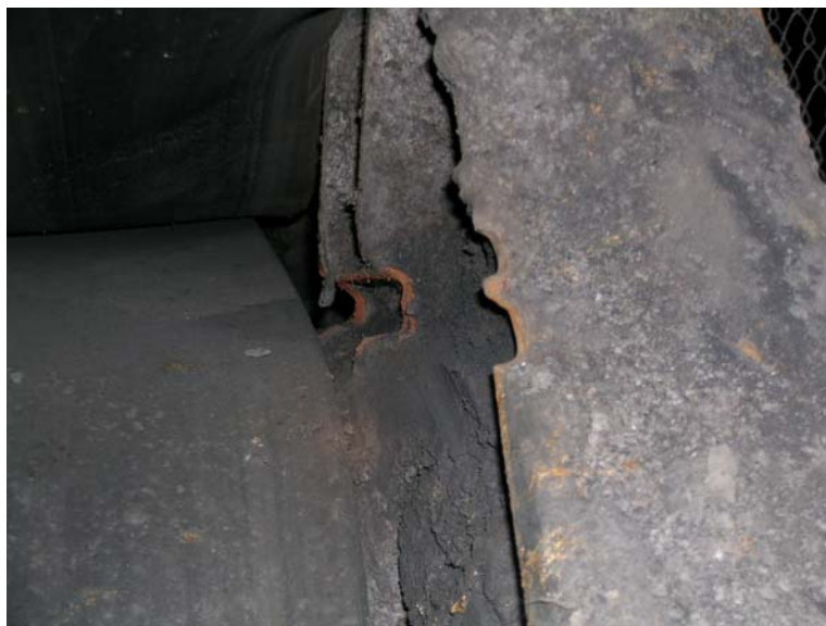
Figure 13. Grooves cut into the rear frame assembly.
