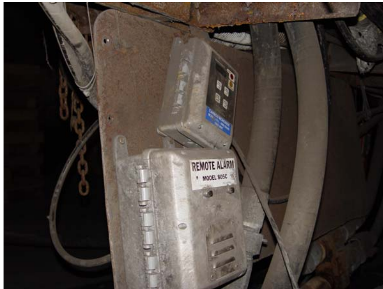
Figure 10. Remote alarm unit in headgate area on longwall section.
