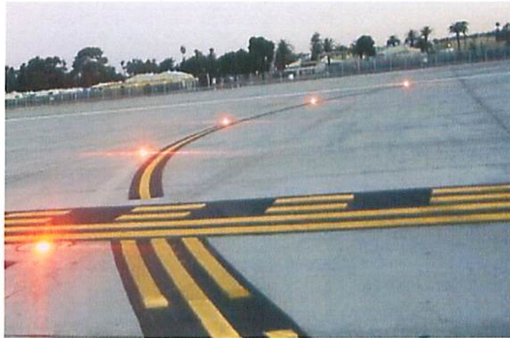
Figure 4: Runway Entrance Lights
