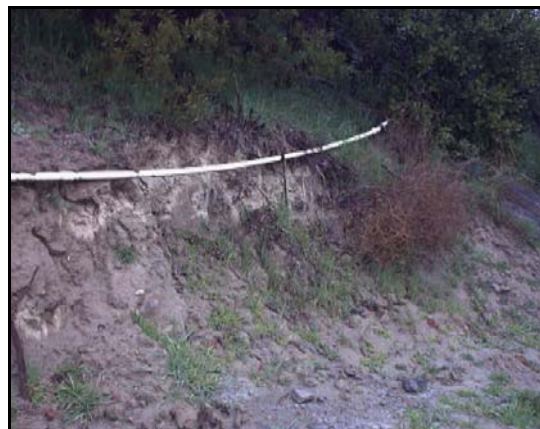
Photograph 2-5. Erosion just off NMCS D Property along its Southeastern Border
