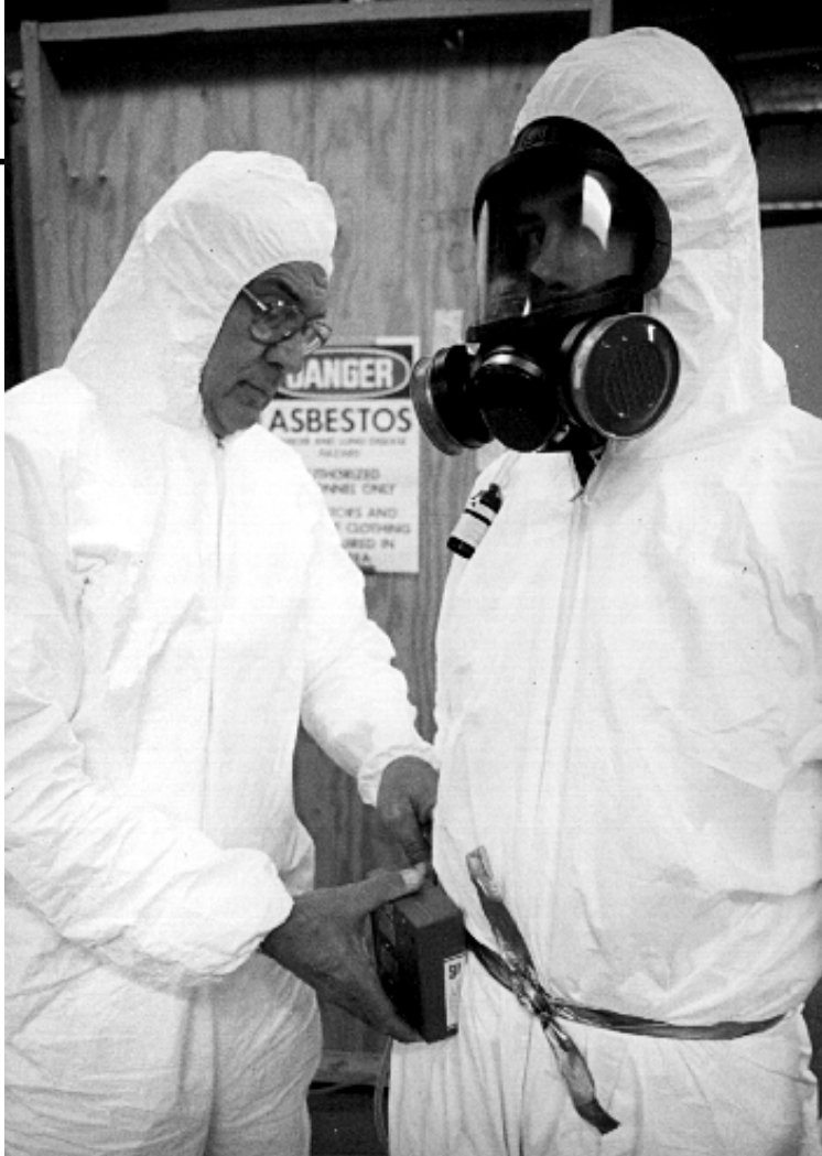
Education Center students at Niagara County Community College prepare to go through the personal decontamination chamber before entering the work area to remove asbestos.
