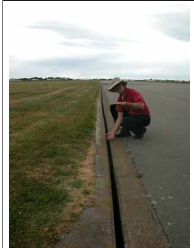
Earthworms crawling onto runways after heavy rains can be a strong attractant to gulls and other birds. This runway in New Zealand uses slit drains to block worms from reaching the runway. Other options include brush-sweeping runway edges to remove worms and deploying extra personnel to disperse gulls. As of 2005, there are no chemicals registered in the USA to control earthworms (photo by R. A. Dolbeer, USDA).
