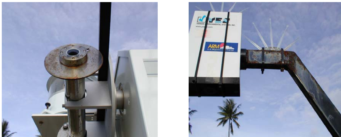
Figure 3. Examples of instrument corrosion.
