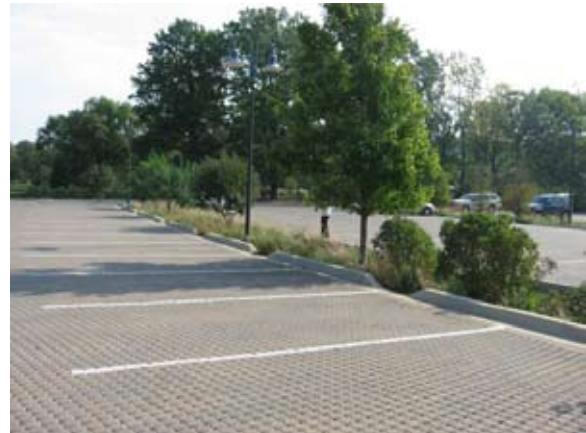
Figure 4-18: Pervious pavers in a parking lot. Any overflow from the pervious pavers drains into a swale.
