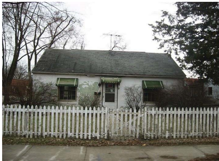
Figure 1: One of the hundreds of homes damaged by the flooding in 2008. (Source: EPA)
