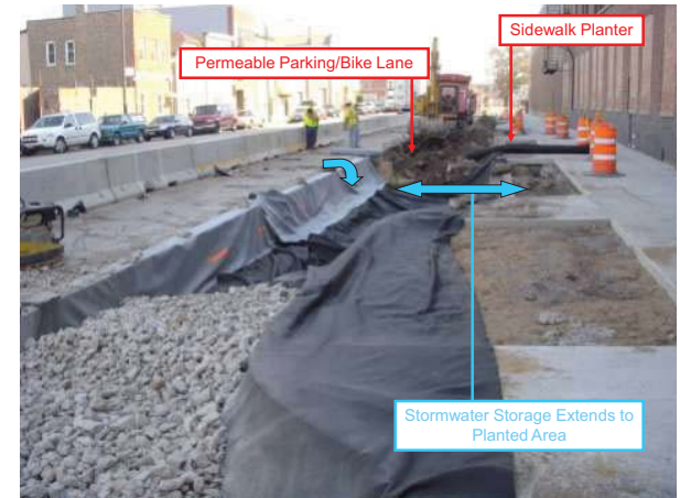
Figure 59: Cermak Road during construction of permeable parking, stormwater storage, and sidewalk planters.
