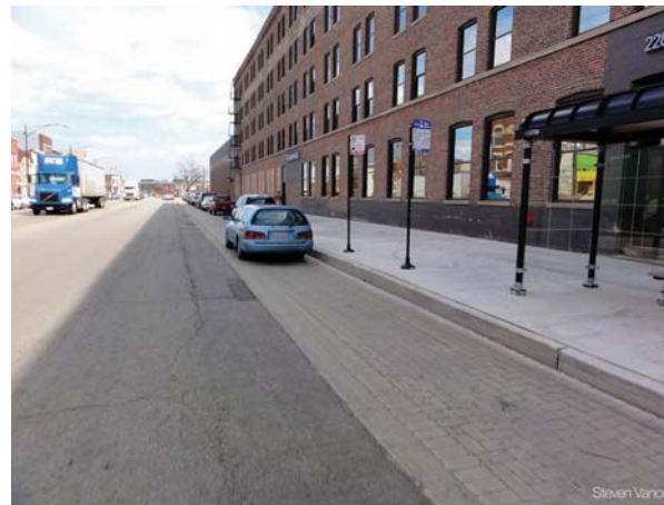
Figure 60: Permeable pavers mark a bike lane and parking area. The pavers contain a special compound to absorb nitrogen oxides.
