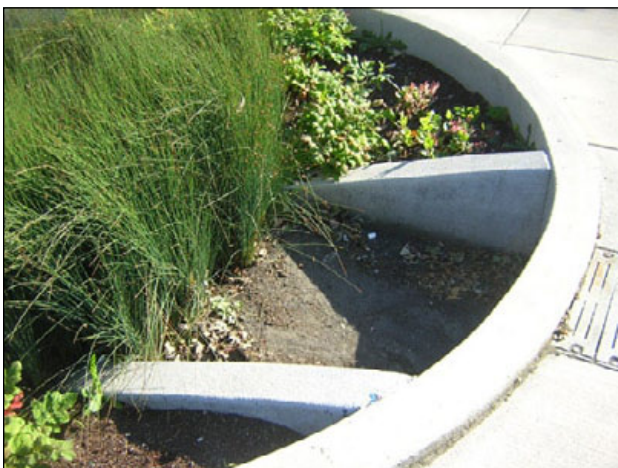
Figure C-25. Sediment forebay in a street infiltration garden.
