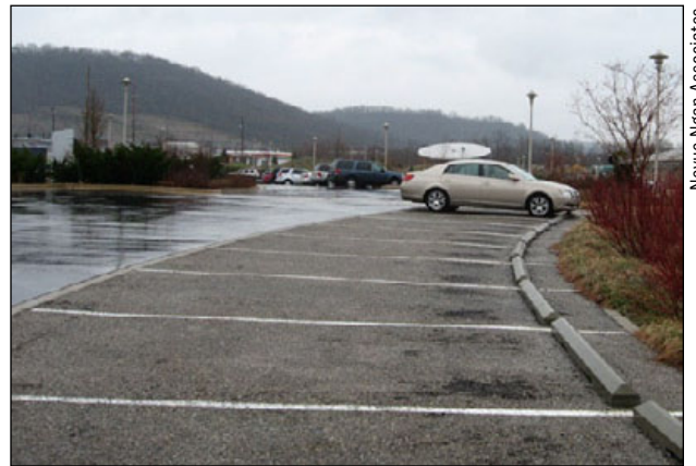
Figure 45. There is no wet sheen on the pervious asphalt in the parking stalls in this parking lot, compared to the conventional asphalt paving in the drive aisles.
