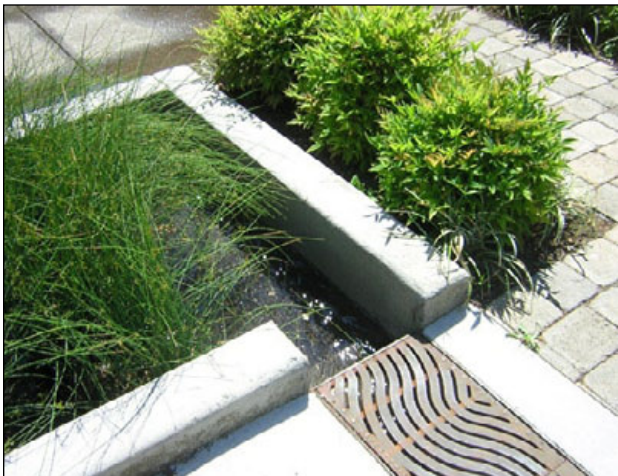
Figure C-24. Sediment forebay in a street planter.
