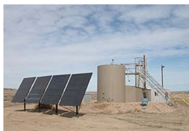
Solar-powered pump station in Wyoming
