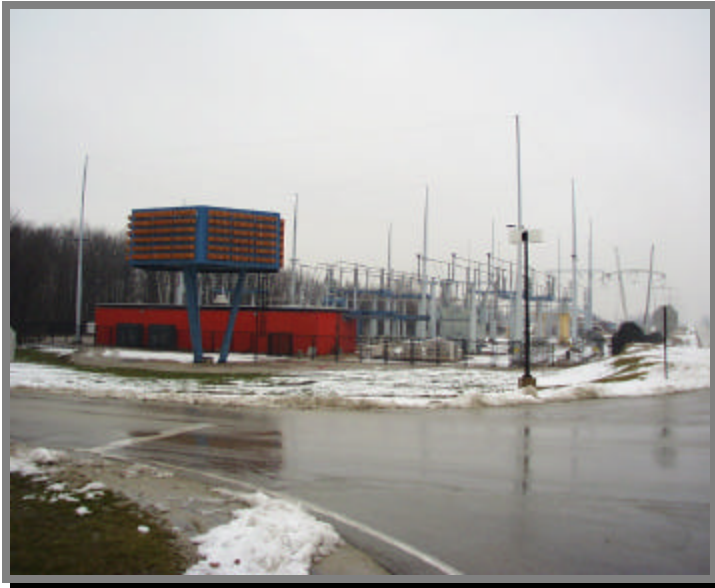
Figure 2-11: Substation near Wilson Hall
