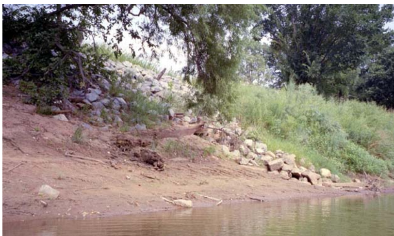
Riprap stabilizes the stream bank where the existing Anadarko Aqueduct crosses under the Washita River.
