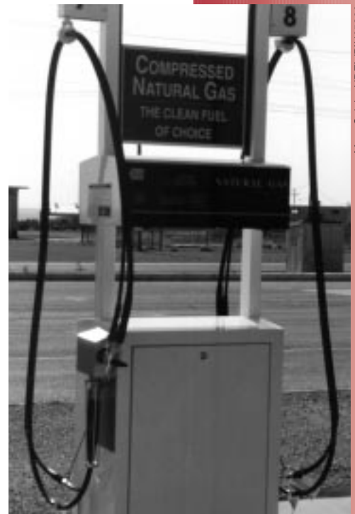
This compressed natural gas station at White Sands Missile Range is one of 14 energy-saving projects under an area-wide contract developed by FEMP in New Mexico that will save the base more than $2 million per year.
