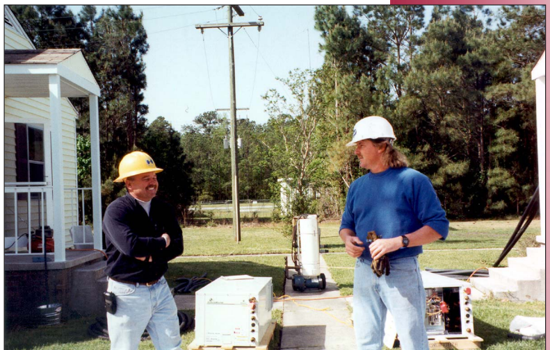
GHPs ready to install and installation crew in Midway Park housing area.
