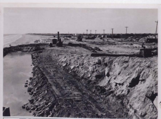
CORPS OF ENGINEERS U.S. ARMY GALVESTON DISTRICT Looking N. from Sea Wall at 61st St. showing excavation preparation for driving timber bearing pile. 12 Dec 1951 Truttl & Thomson, Inc. Cont. No. Da-41-56, base-1152 Pict. 30 Aug. 1951 8 x 8 Photo Photo 9
