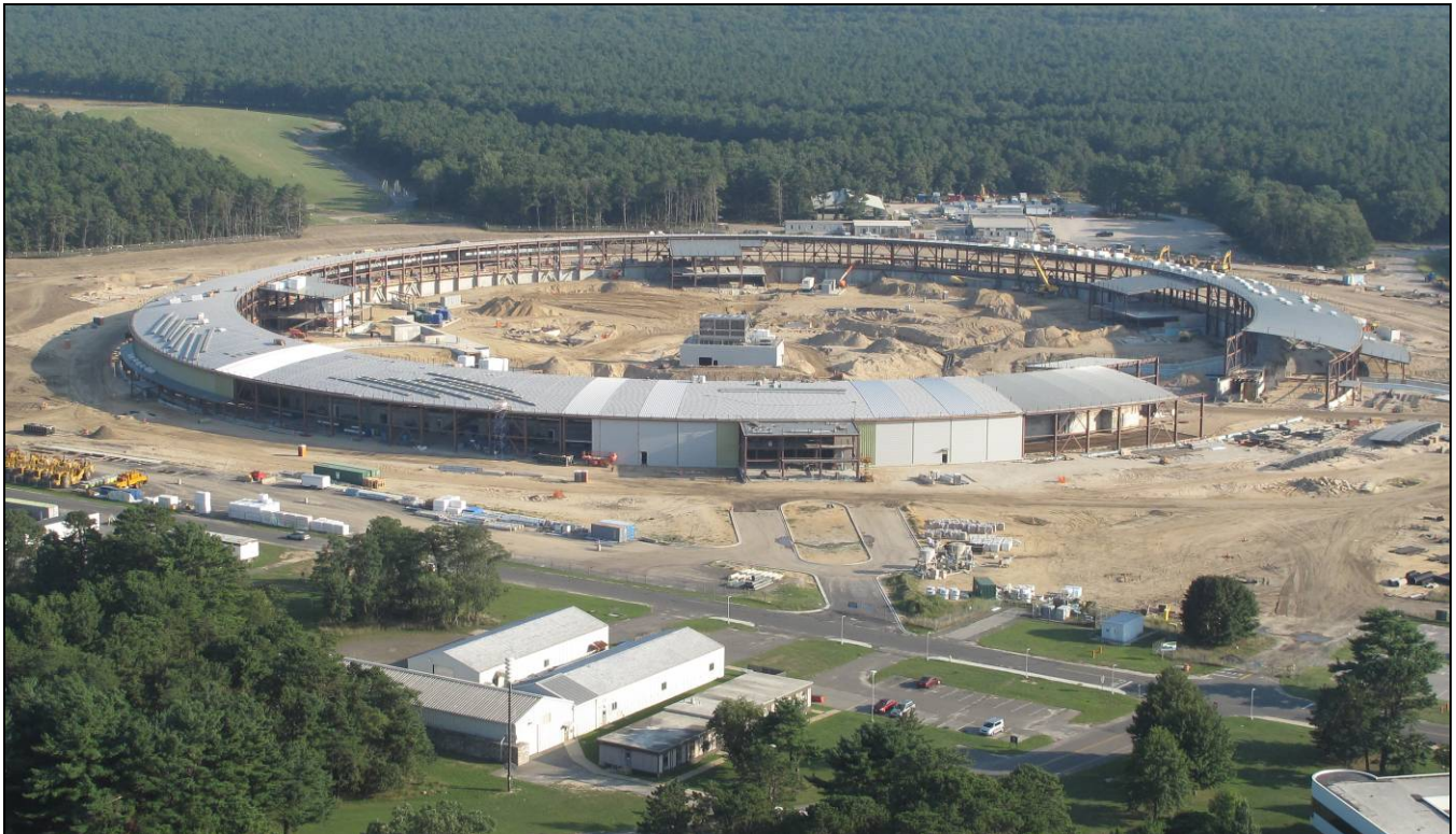
August 31: Progress on conventional facilities continues, with siding and roofing installation most visible in this photo.
