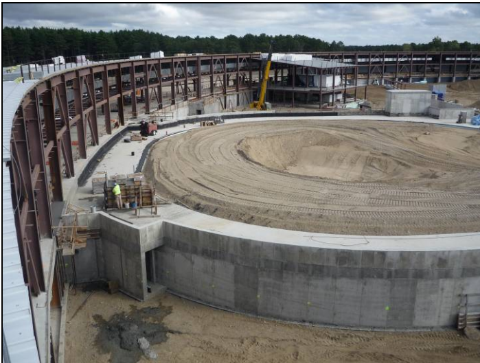
Figure 6. Waterproofing of the booster tunnel roof begins. Note also that backfill operations at the booster tunnel are in progress.
