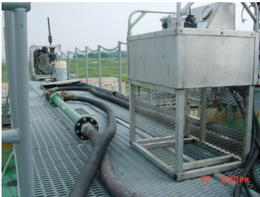
Figure 6. In-line mixer on deck connected to discharge hose just before recovery tanks.
