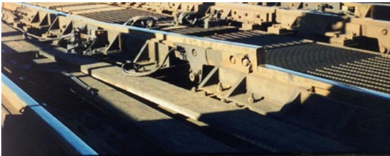
Figure 2 — Looking west at the west end of track 1. The heel of the miter rail is elevated about 5 inches above the running rail, creating a ramp for the left side trucks of any eastbound train. (Photograph taken on the day of the accident after removal of the derailed equipment.)
