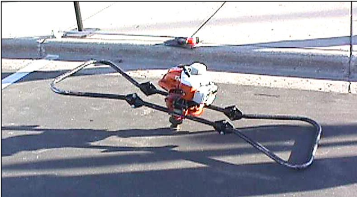
Figure 3. The “anchor cranker” auger used to install the anchor that ruptured the pipeline
