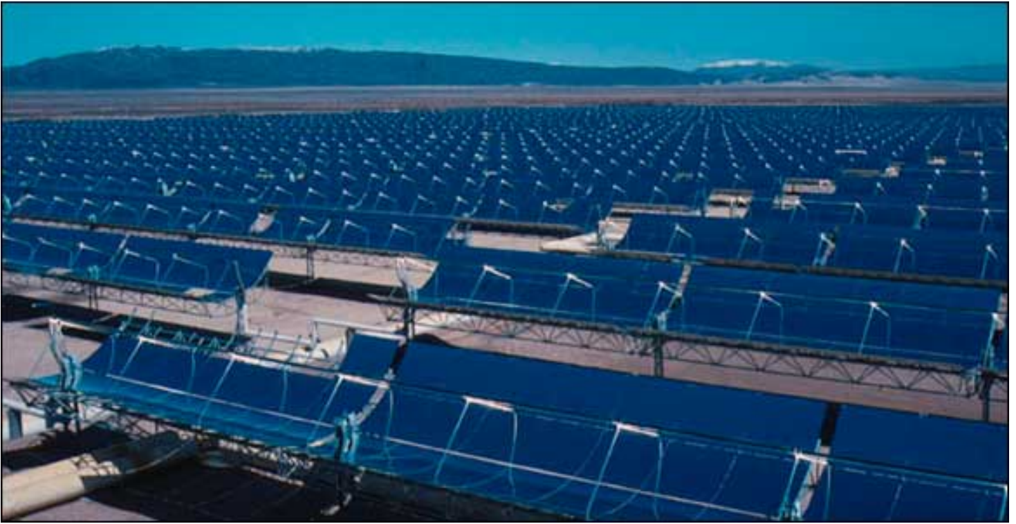
Solar Power Plant
