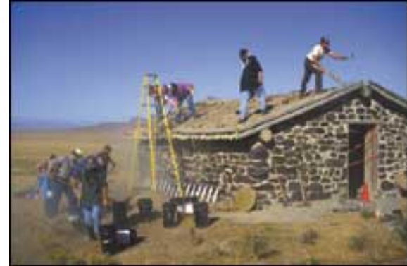
Recreational improvements (volunteers repairing the roof of a Pony Express Station), West Desert, UT.
