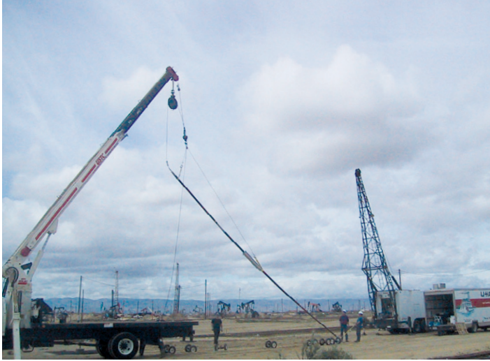
Figure 22. The Geo-BILT logging tool being deployed in an oil field
