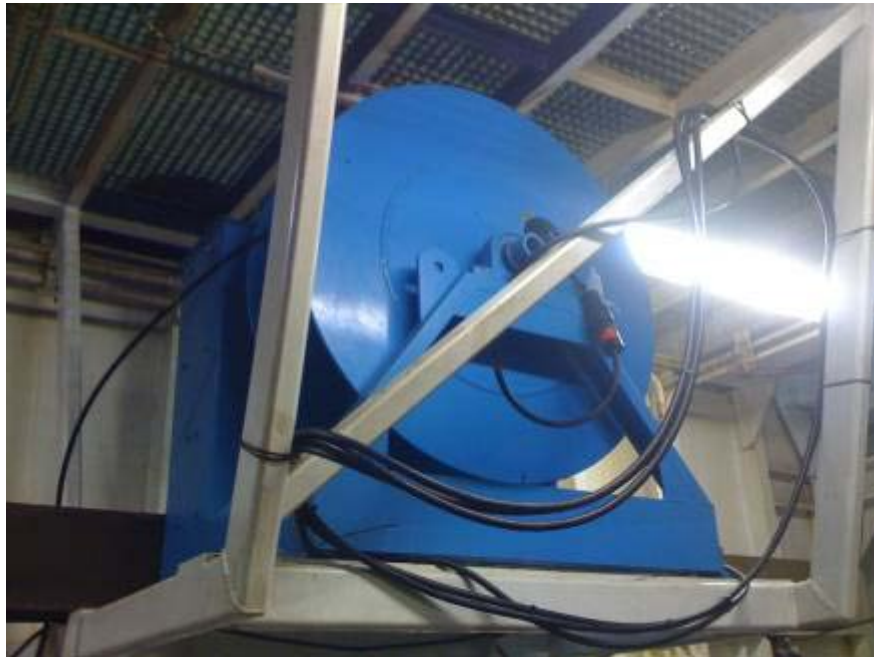
Figure 3. Hydrophone cable on winch
