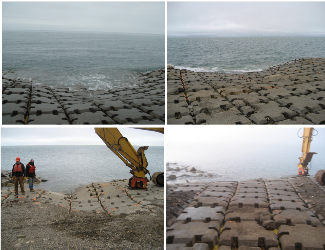
FIGURE 2.8. Before and after the 2008 repairs at the north side swale area (A=before; B=after) and at the southeast side swale area (C=before; D=after).
