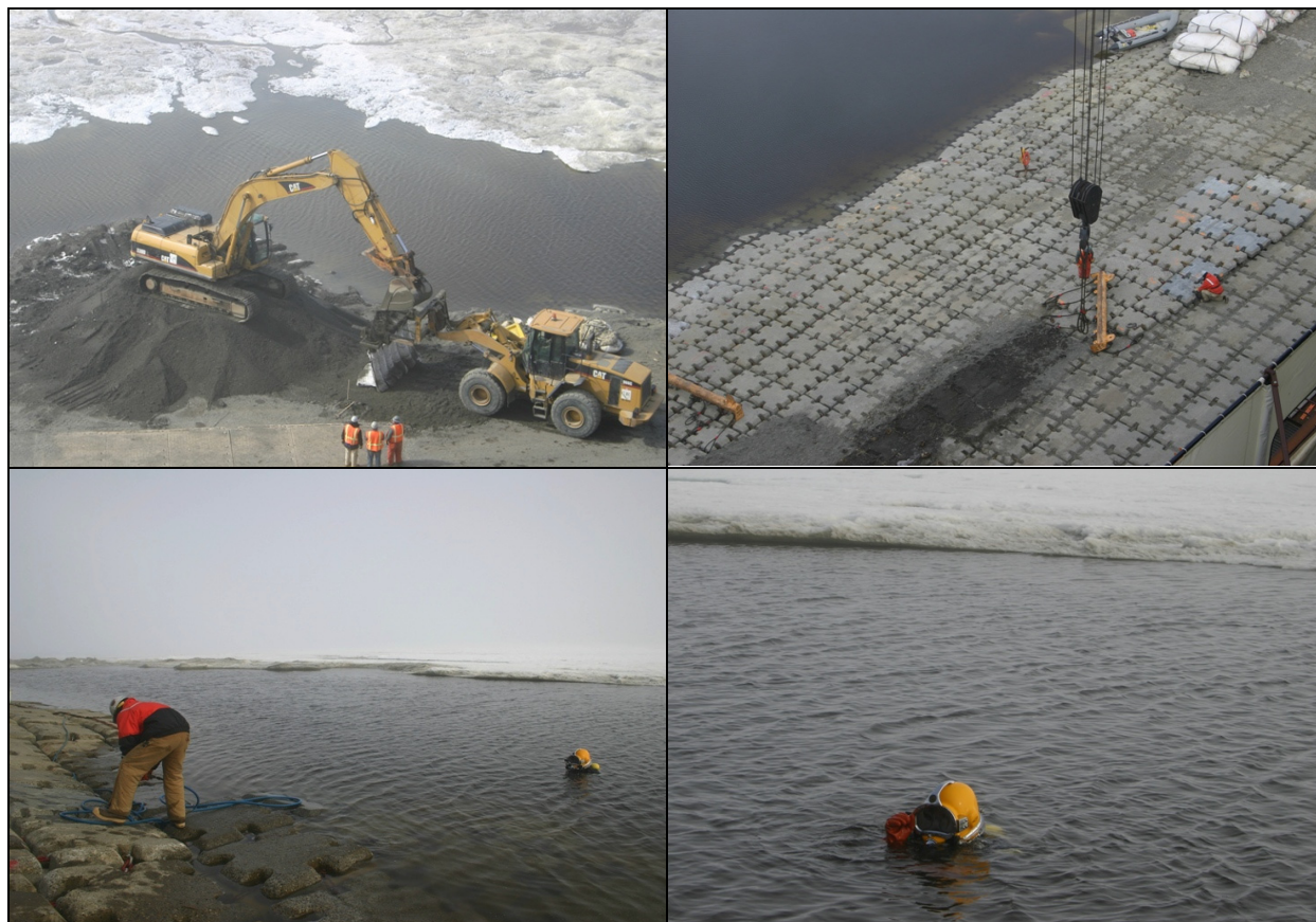
FIGURE 2.9. Block system and fabric repair (above left and right) and diver repair work (bottom left and right) at Northstar Island in 2009.
