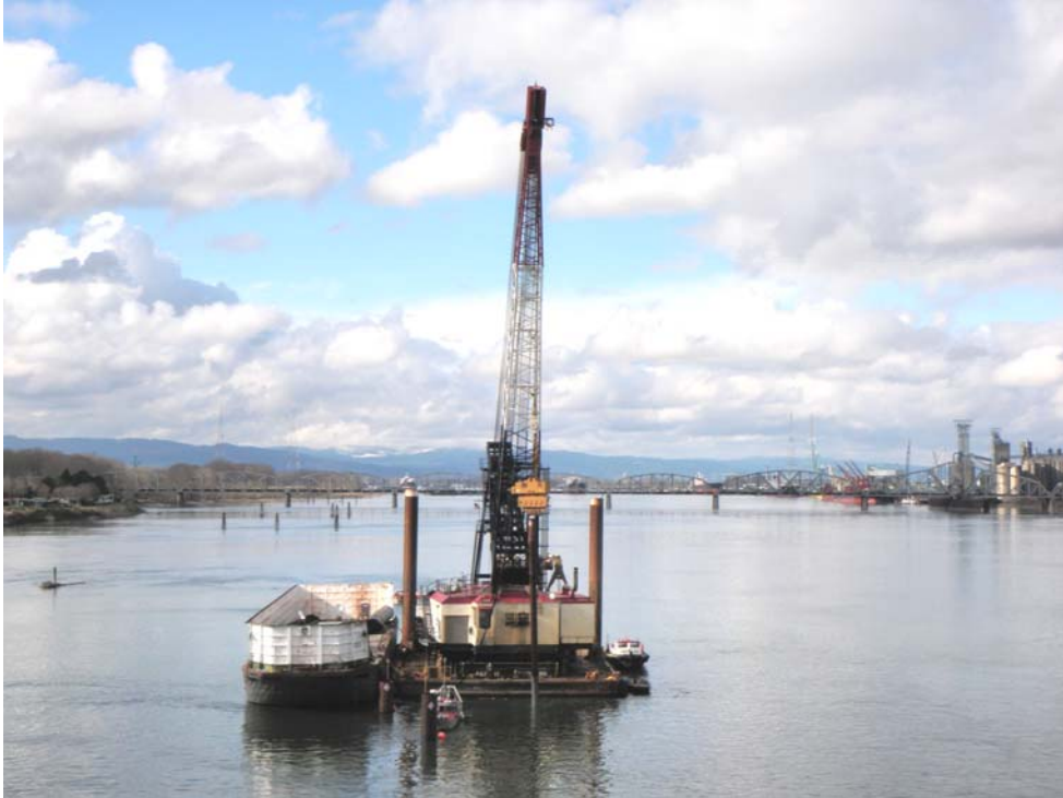
Photograph 1. Typical view from the I-5 bridge facing downstream toward test pile activities.
