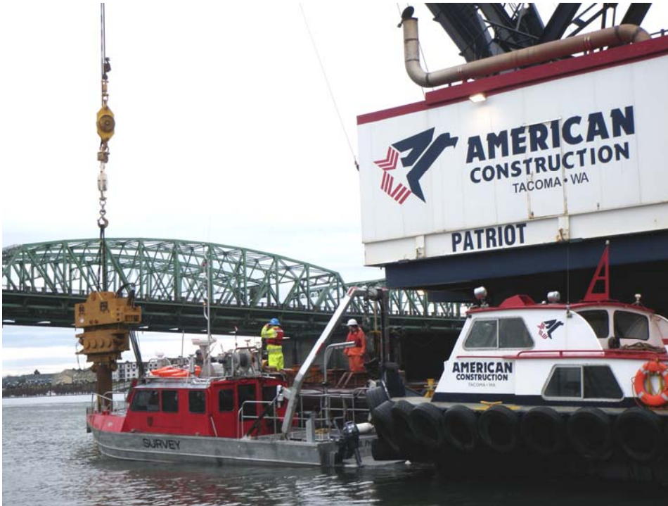
Photograph 2. Monitor (shown in yellow) on the work barge scans for marine mammals during vibratory pile activities.
