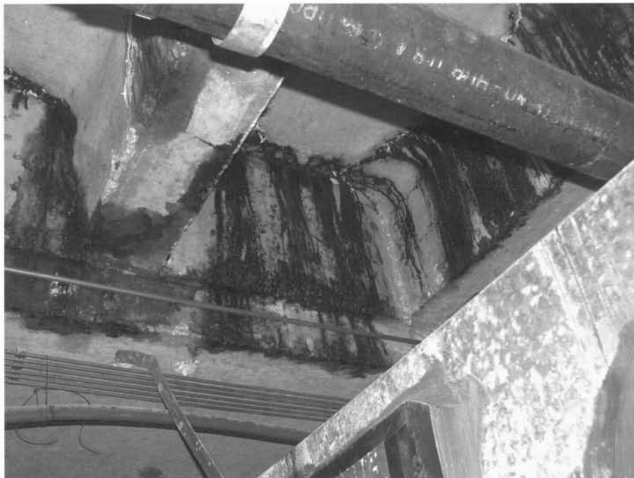
Photograph of the ceiling of the basement room where the dean's office records were stored showing the leakage from the morgue. Photograph courtesy of Nina Stoyan-Rosenzweig.
