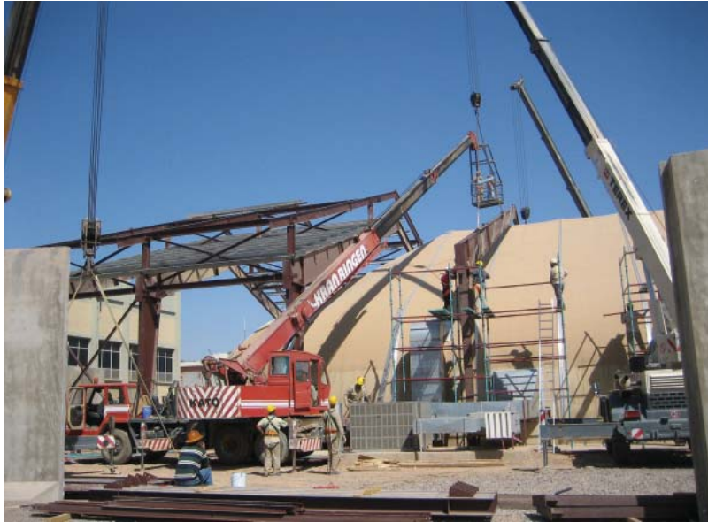
USACE has managed the construction of overhead protective covers at more than 20 locations in Iraq since 2005 and this quarter awarded a $55 million contract for covers at three additional locations. (USACE photo)
