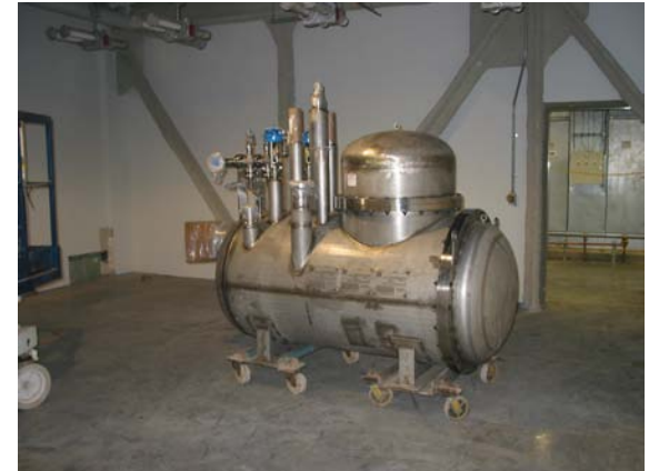
He/H2 Heat Exchanger Module
