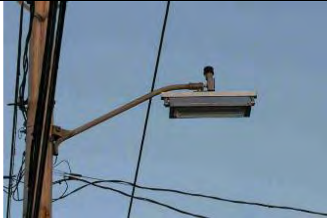
Figure 7. Fluorescent luminaire with drop lens
