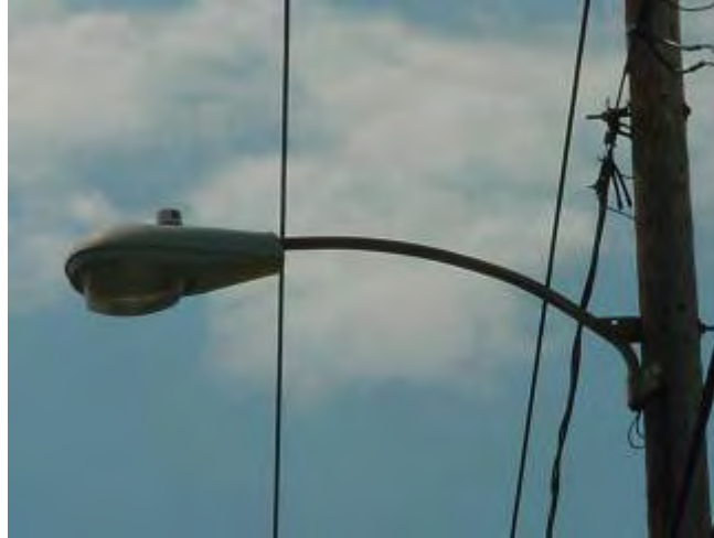
Figure 3. Existing HPS luminaire
