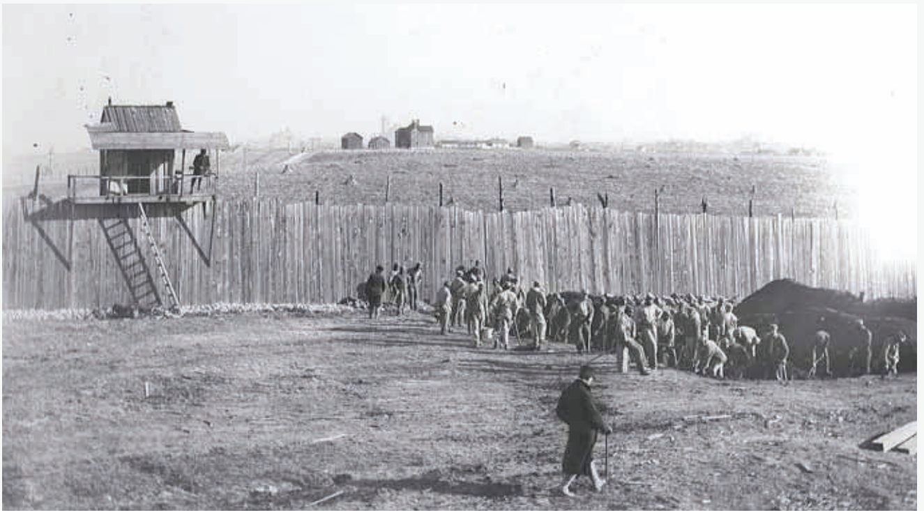
Inmates at Fort Leavenworth begin work on the foundation for the new U.S. Penitentiary in 1902.
