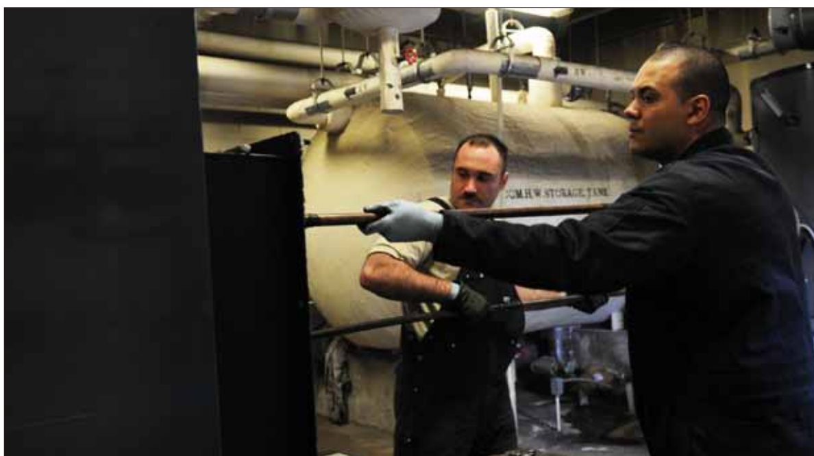
Airman 1st Class Jonathan Pears, left, and Staff Sgt. Alexander Angel, 8th Civil Engineer Squadron heating, ventilation, air conditioning and refrigeration technicians, clean a boiler Feb. 15, 2012, at Kunsan Air Base, Republic of Korea. The pair was named the "Pride of the Pack" for the 110 hours of overtime they put in to ensure Airmen had heat and hot water. (U.S. Air Force photo by Senior Airman Brigitte N. Brantley)
