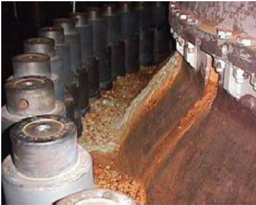
Rod Rusty Boric Acid Deposits on Vessel Flange (12RFO)
