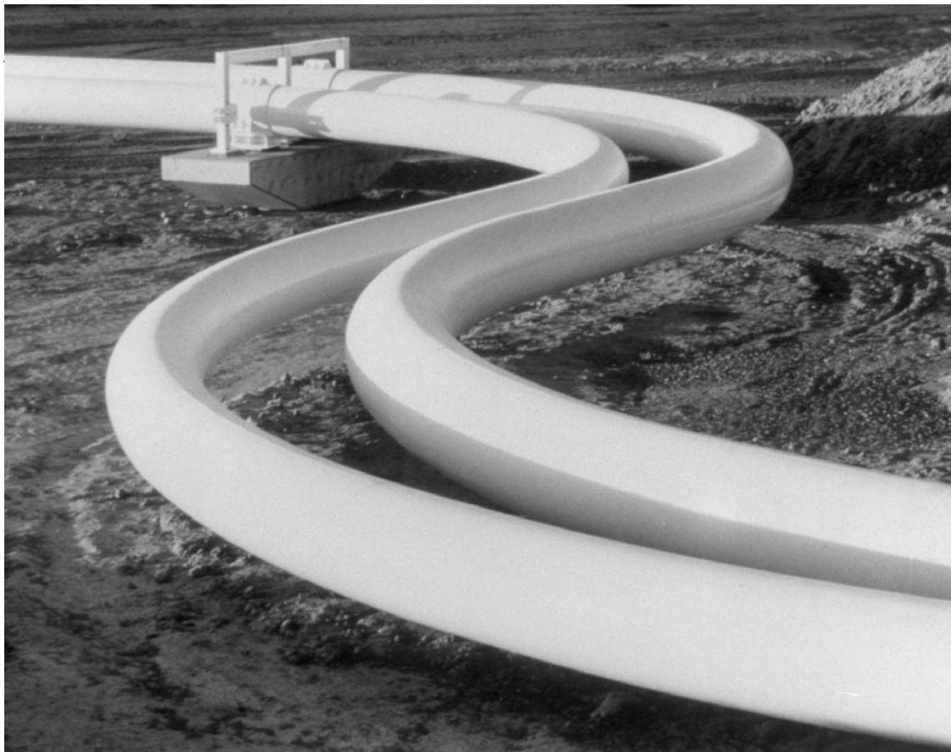
Natural gas pipeline, El Paso County, Texas. Source: U.S. Department of Energy.
