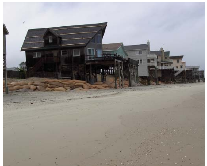
Photo 21. Geotextile sand bags along the beach in Nags Head, North Carolina. Although the homes were on pilings, the geotextile sandbags were needed to protect the septic tanks. (June 2003). [Photo source: ©James G. Titus, used by permission].
