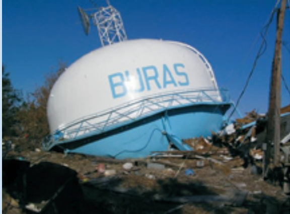
The collapsed water tower in Buras, Louisiana, attests to the fury of Hurricane Katrina as she first made landfall in the lower Mississippi Delta. Photo: Lewis Kozlosky
