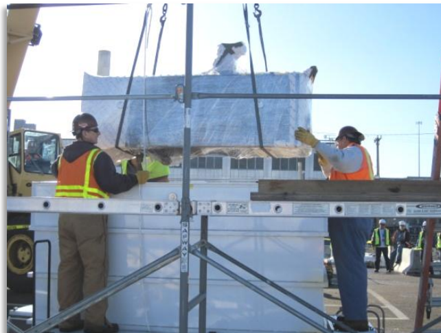
PFP crews load a glovebox into a Standard Large Box 2 (SLB2) container
