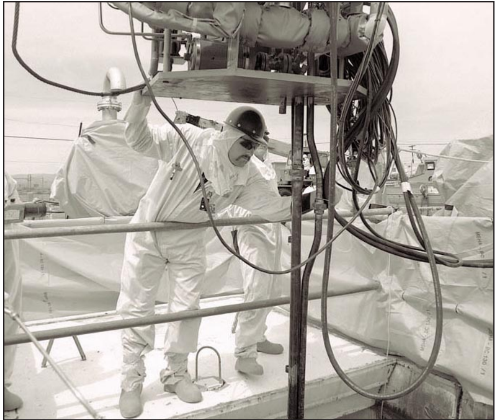
Workers install the pump for S-103, one of the most recent single-shell tanks to enter the pumping phase.
