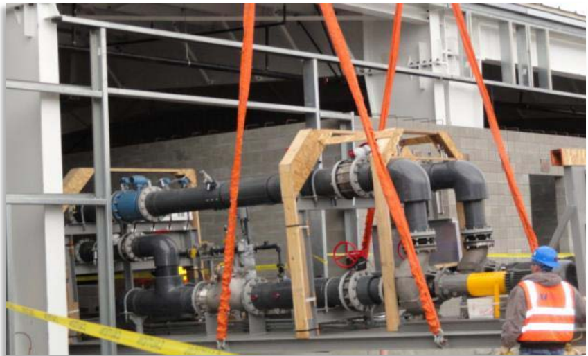
In mid-March a skid arrived for installation in the Bio-Process Building of the 200 West Groundwater Treatment Facility.
