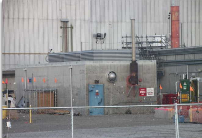
The first of six buildings to be demolished at the PFP vault complex
