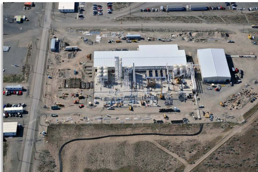
Aerial view of the 200W Groundwater Treatment Facility Biological and Radiological Process Buildings
