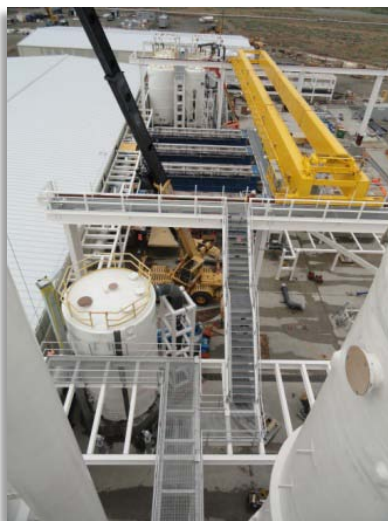
200 W Groundwater Treatment overhead crane
