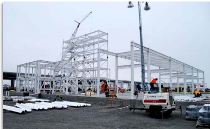
Ongoing structural steel erection of the Stair Towers for the Aerated Sludge Tank and Air Stripper at 200W Groundwater Treatment Facility
