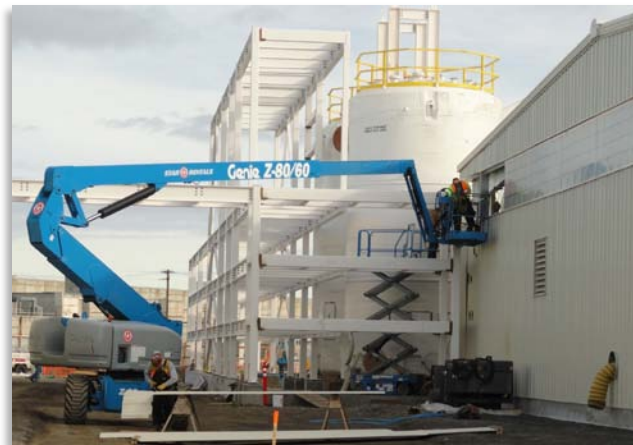
Construction of the Bio-Process Building for the 200 West Groundwater Treatment Facility continues.
