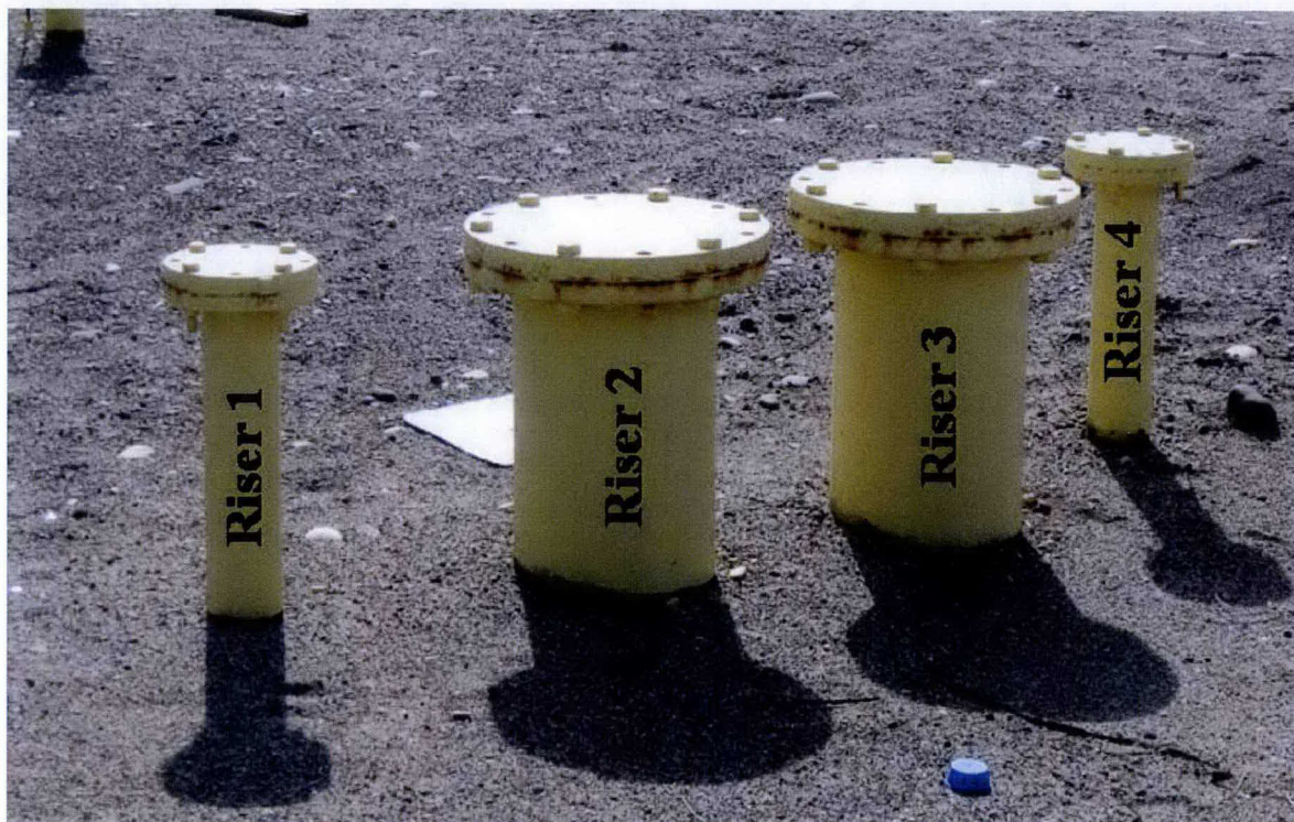
Figure 5. Catch Tank Risers 1 Through 4.
