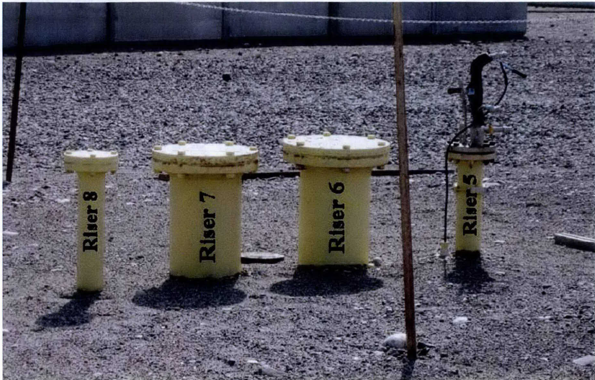
Figure 6. Catch Tank Risers 5 Through 8.
