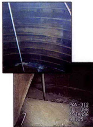
Ripped and buckled floor liner in Tank A-105
