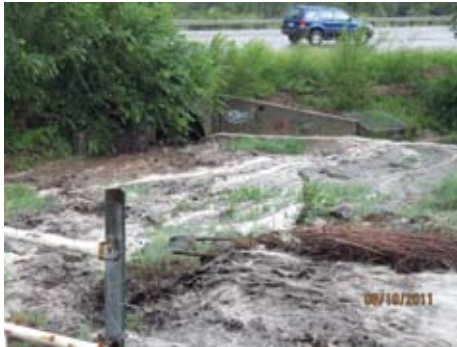
Same drain - flow during storm
