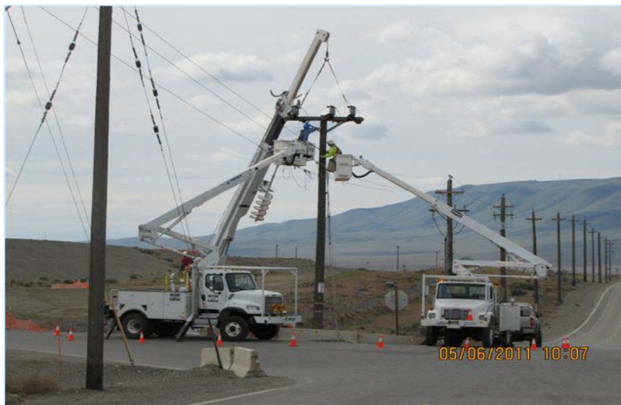
Electrical Utilities crews relocate pole G507 at Environmental Restoration Disposal Facility (ERDF) Entrance
