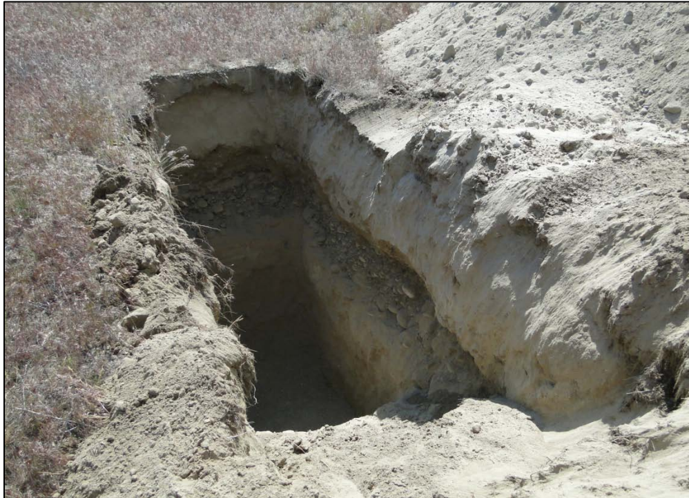
Project L-691 – “Test Holes to confirm soil characteristics for the Lagoon Project”
