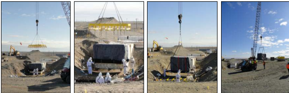
Crane & Rigging performing critical lifts in support of CH2M HILL Plateau Remediation Company (CHPRC) Transuranic (TRU) Retrieval.
