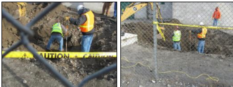
Teamsters and Heavy Equipment Operators repair an underground water leak at B Reactor
